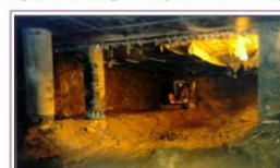
Fig. 13. «The Alfa-Arbat-Center» multifunctional complex in Moscow. Excavation in the 3rd tier of the pit under the parking-garage western half 2nd-storey ramp.
