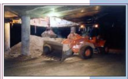
Fig. 12. «The Alfa-Arbat-Center» multifunctional complex in Moscow. Hitachi W130 motor loader transporting truck to temporary erection opening while excavating the 2nd tier of the pit. Truck is brought to the surface using Hitachi EX300-5 clamshell excavator and loaded into dump trucks.
