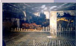
Fig. 19. «The Alfa-Arbat-Center» multifunctional complex in Moscow. Completing excavation of the 5th tier of the pit near the erection opening.
