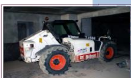
Fig. 16. «The Alfa-Arbat-Center» multifunctional complex in Moscow. Facing materials transported over the ramp to the 3rd storey with small-size loaders while excavating the 5th tier of the pit.
