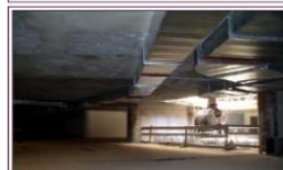
Fig. 17. «The Alfa-Arbat-Center» multifunctional complex in Moscow. Installing ventilation and fire-fighting permanent systems at the 2nd storey while excavating the 5th tier of the pit.
