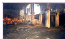
Fig. 15. «The Alfa-Arbat-Center» multifunctional complex in Moscow. Excavation in the 4th tier of the pit in the parking-garage eastern half ramp area.
