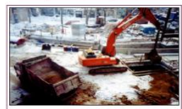
Fig. 11. «The Alfa-Arbat-Center» multifunctional complex in Moscow. Hitachi EX300-5 clamshell excavator working through temporary erection opening and bringing truck to the surface to be loaded into dump trucks while excavating 2nd tier of the pit.
