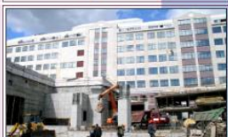
Fig. 18. «The Alfa-Arbat-Center» multifunctional complex in Moscow. Completing construction of the extension to the main building. Erecting structures of the third stage construction package over the underground parking-garage eastern half while excavating the 5th tier of the pit.
